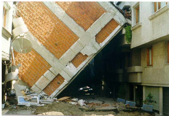
Figure 1.7: Manifestations of liquefaction in Adapazari (Kocaeli Earthquake 1999)
